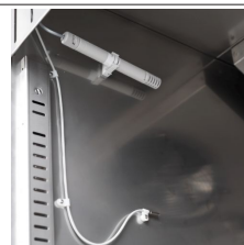
Humidity control with electronic probe
