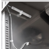
Humidity control with electronic probe
