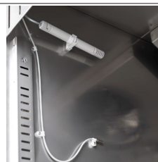
Humidity control with electronic probe
