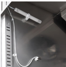
Humidity control with electronic probe
