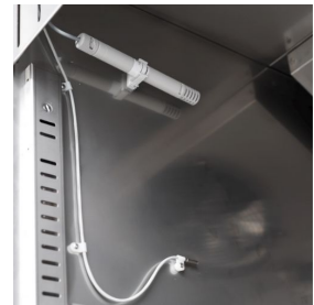
Humidity control with electronic probe
