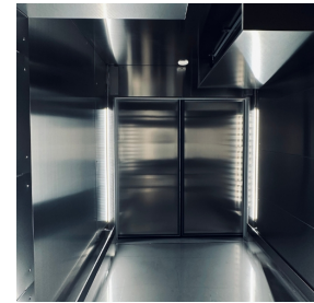
Internal lighting with LED lights
